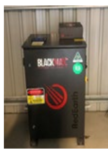
(off-grid solar battery)
